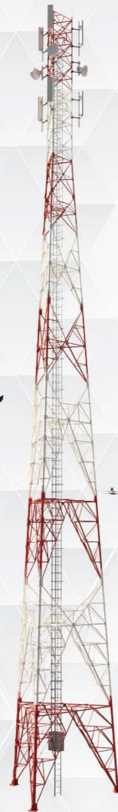
Lattice Tower p101
